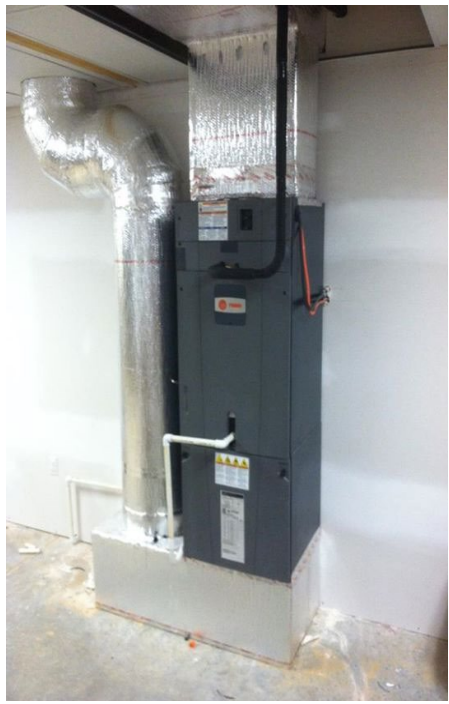
Central Air Handler
